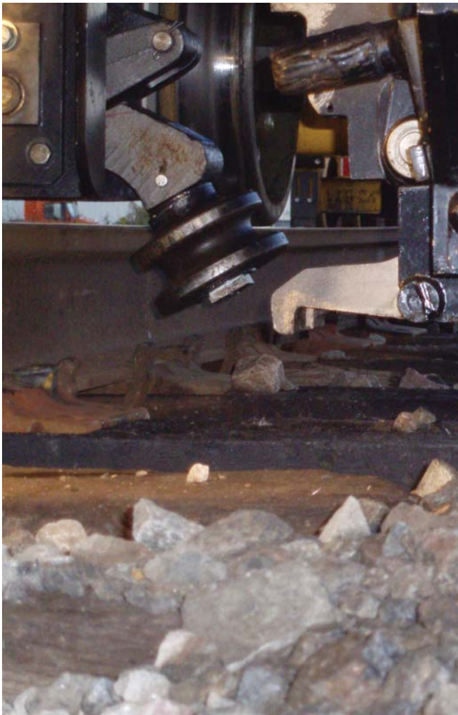
Rail jacks raise the rail while the finger assembly inserts and positions the plate.
