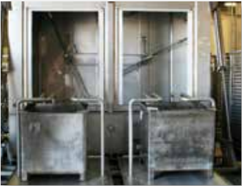
Synchronized rotating spray arms clean the vats' interior and exterior
