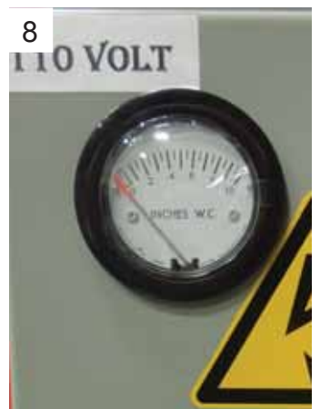
8 Monitor the Minihelic pressure gauge while adjustment to achieve the desired setting. If the Minihelic pressure gauge stays at 6" - 7" H 2 O" and pulsing does not directly improve the differential pressure, replace your filters.
